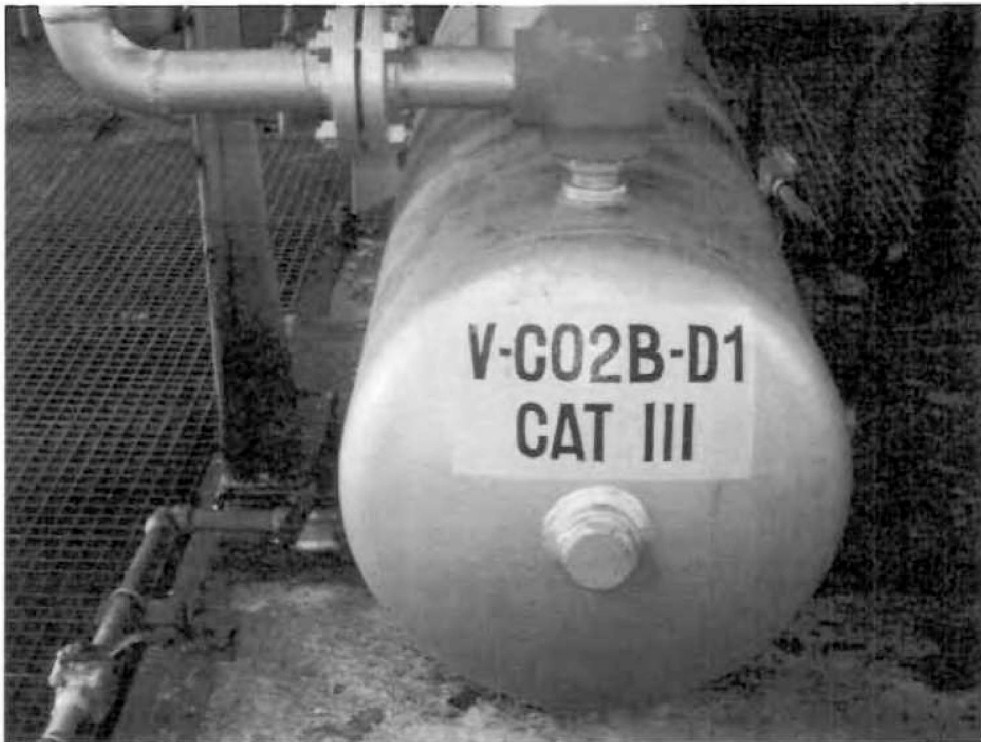
Nº75 - C-02A/B/C – Vaso do Compressor – HSE – 2NL2 - (Área: GLP).
